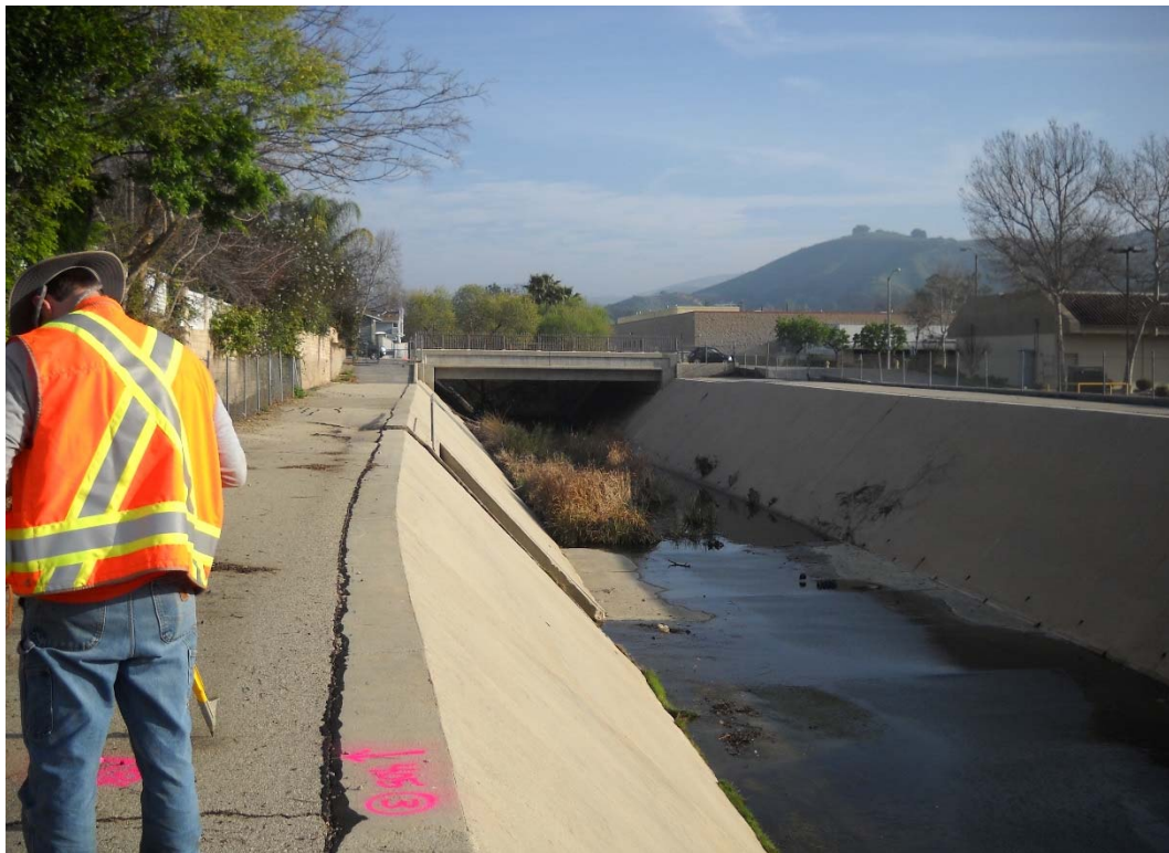
DOWNSTREAM EXTENT OF REACH NO. 33, HEC-RAS RIVER STATION 57+19, UPSTREAM DIRECTION (THOUSAND OAKS BLVD. BRIDGE)
