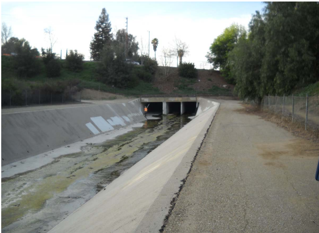
56 FT. UPSTREAM OF HEC-RAS RIVER STATION 39+69, UPSTREAM DIRECTION KANAN RD. CULVERT (UPSTREAM OF REACH NO. 34)
