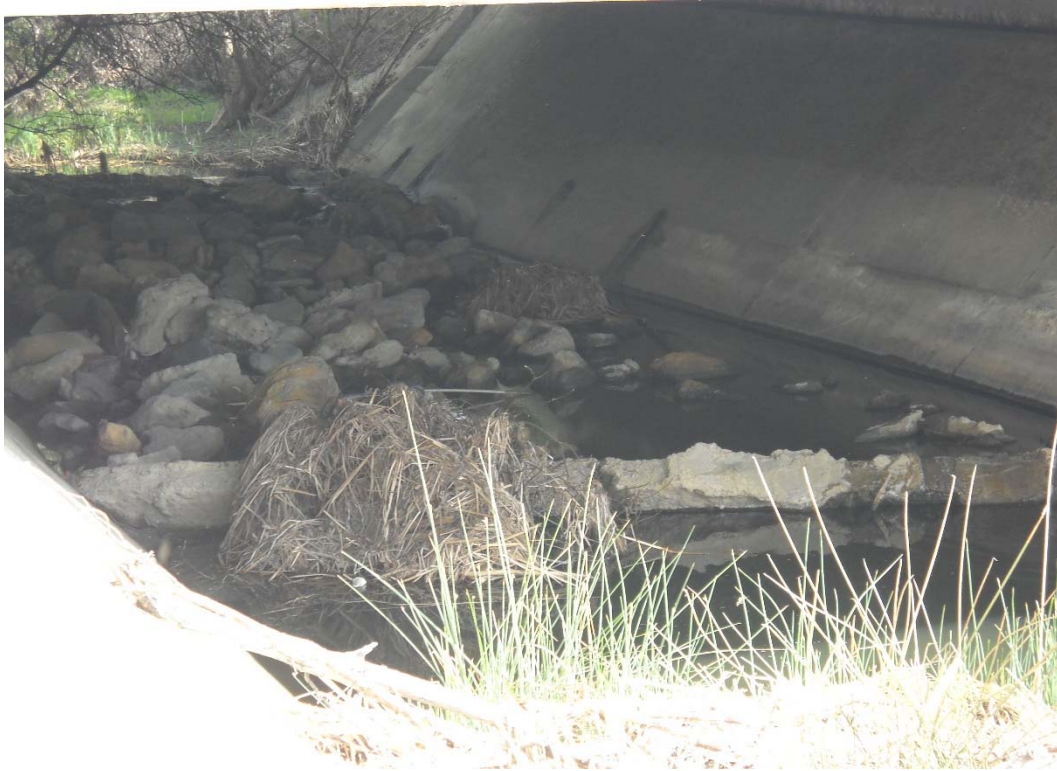
50 FT. UPSTREAM OF HEC-RAS RIVER STATION 58+85, UPSTREAM DIRECTION (BENEATH THOUSAND OAKS BLVD. BRIDGE)
