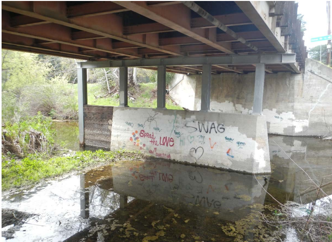
REACH DOWNSTREAM EXTENT, 83 FT. DOWNSTREAM OF HEC-RAS RIVER STATION 12+08, MULHOLLAND HIGHWAY BRIDGE
