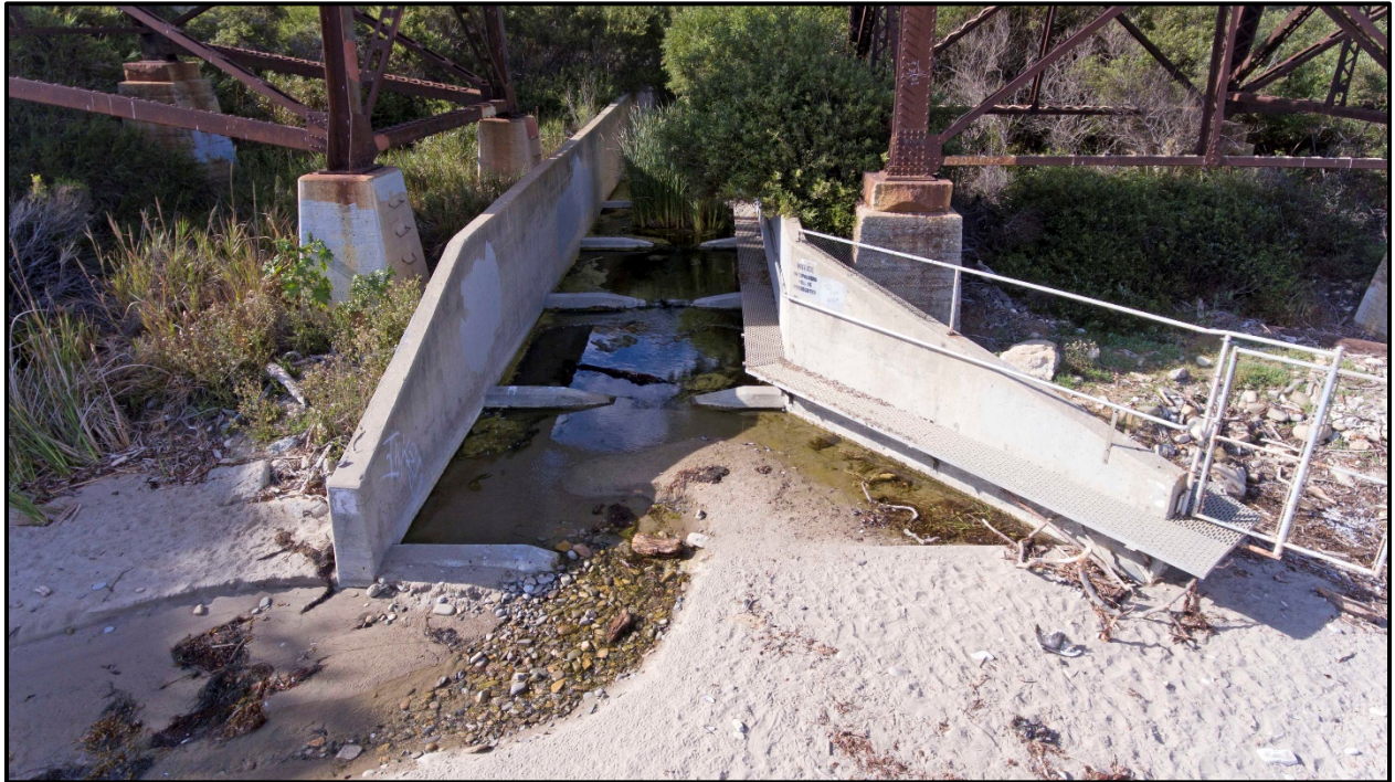
Figure 4-13. Sediment accumulation and vegetation growth in the Arroyo Hondo Creek culvert in Santa Barbara County 2017. This culvert ends at the beach similar to Solstice Creek.
