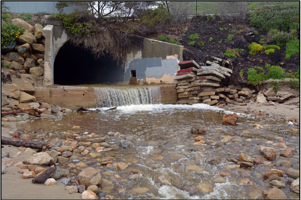
Figure 2-6. Solstice Creek downstream from culvert, February 21, 2017. Recent high flows have exposed underlying cobbles and boulders.
