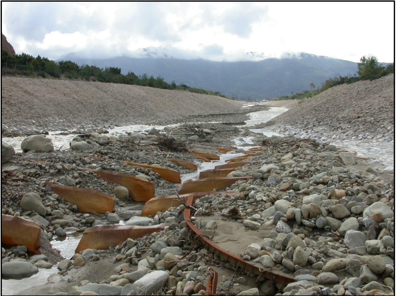
Figure 4-12. Sediment accumulation and pool damage at fish passage structure following 2004/2005 storm events in Santa Paula Creek. The creek bypassed the structure on the right bank (looking downstream).
