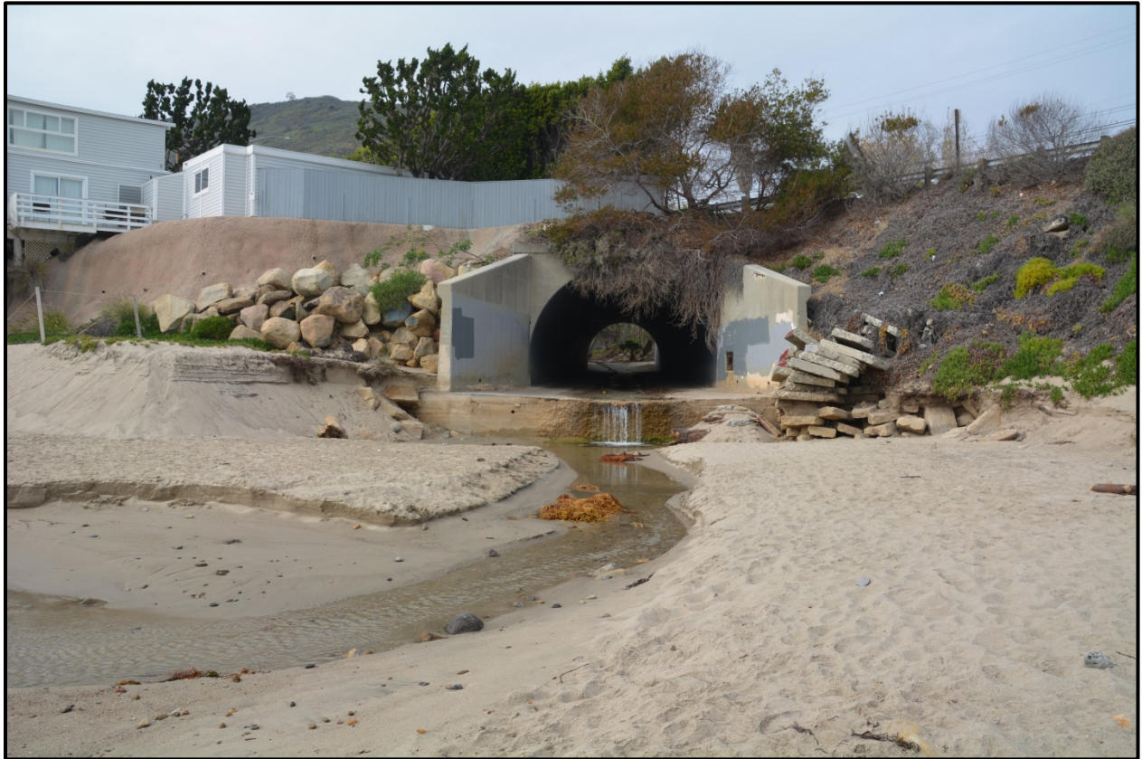
Figure 1-3. Looking upstream towards Solstice Creek Culvert, February 2, 2017. Following storms in late January, there was a four-foot drop at the culvert outlet.
