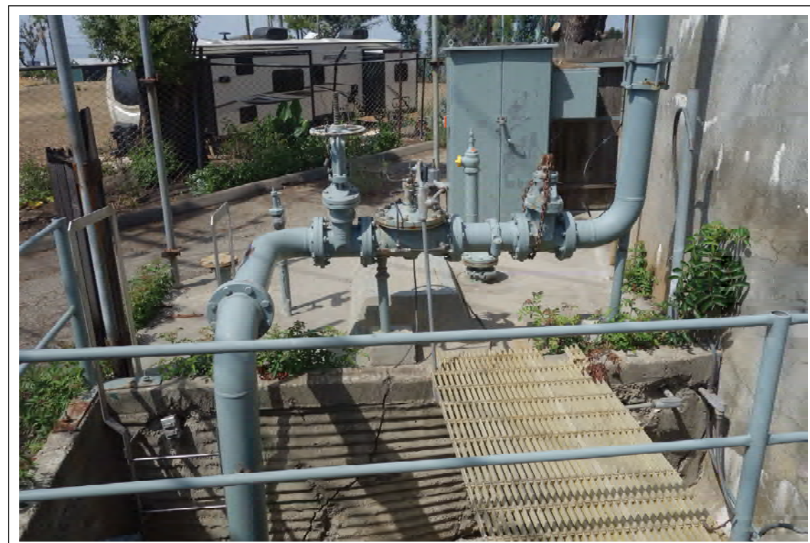
Photo 4: View looking southwest from the southeast part of the site of piping on the southeast side of the tank; the trailer in the background is offsite to the south.
