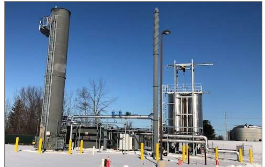
Biogas Upgrading System at the London Facility
