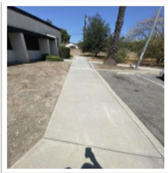
Signage to accessible entrance should be provided.
