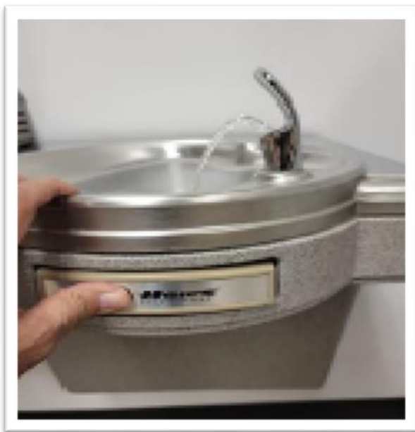
Low water flow at Malibu facility at time of inspection.
