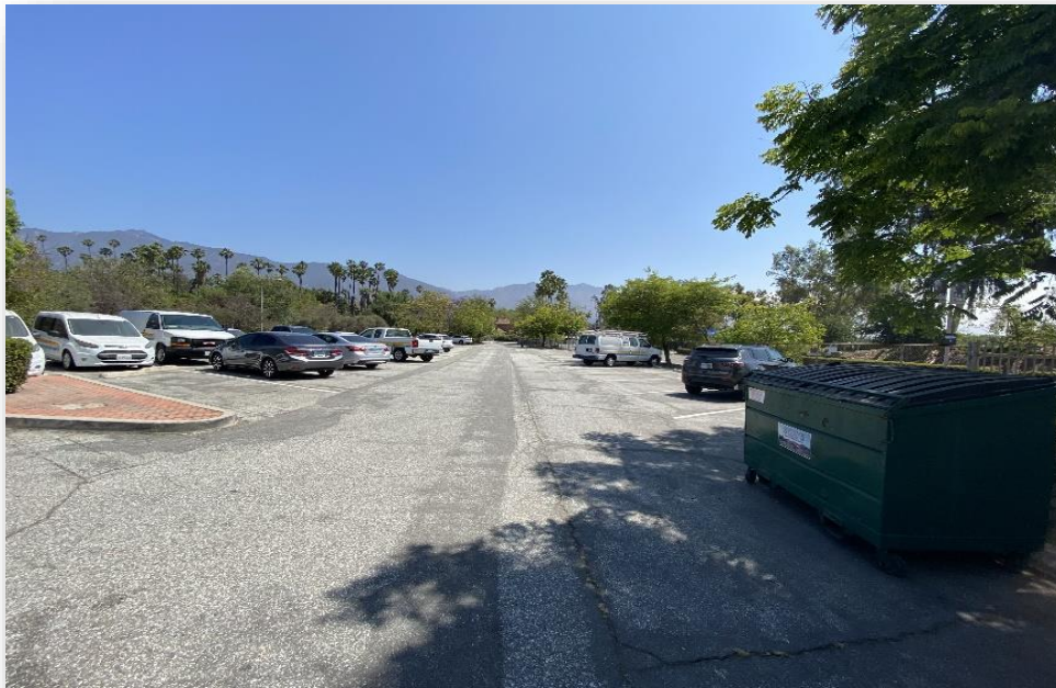
A view of a parking lot with no identified path of travel, and no signage directing users to an accessible entrance
