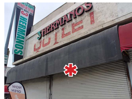
* Poorly maintained cloth awnings
