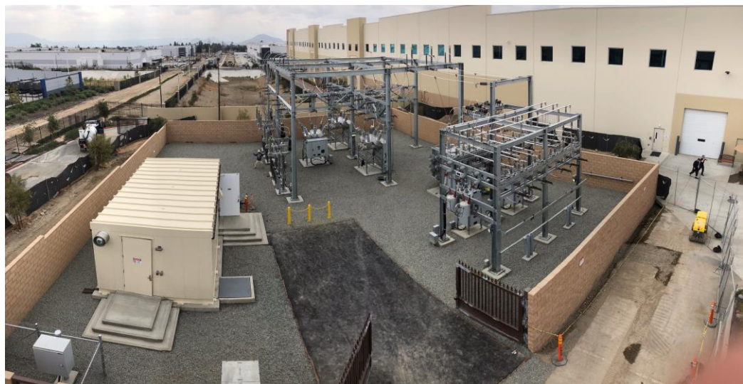
Similar Facility (Medicine Substation would have two transformers)
