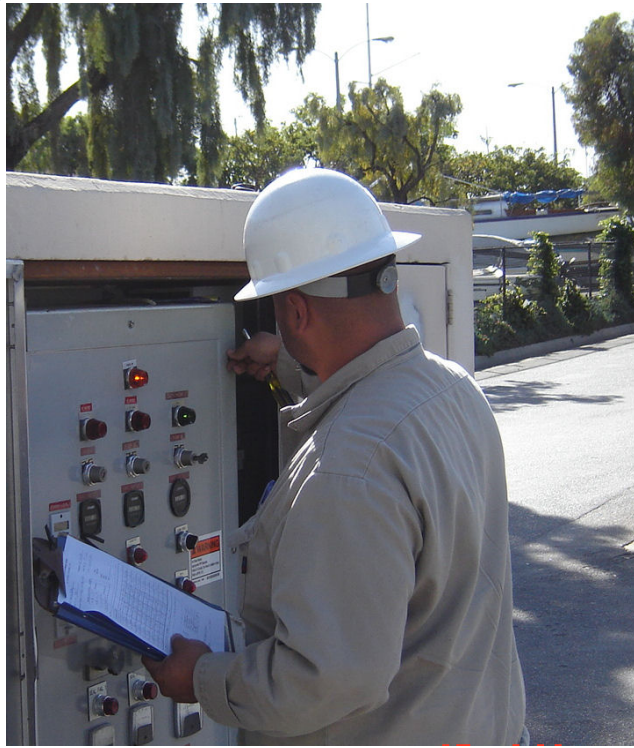
Worker is checking panel for the pump times.
