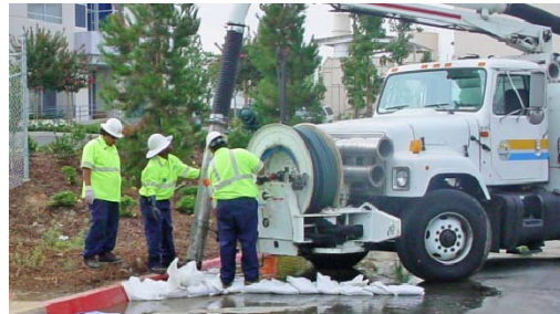
Workers using a hydro vacuum truck to clean up overflow from street surface.
