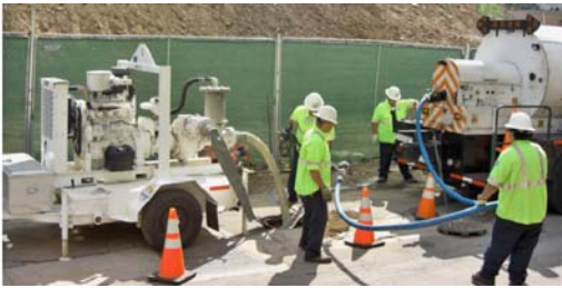
Workers using the rodder truck to clear sewage blockage in a pipe.
