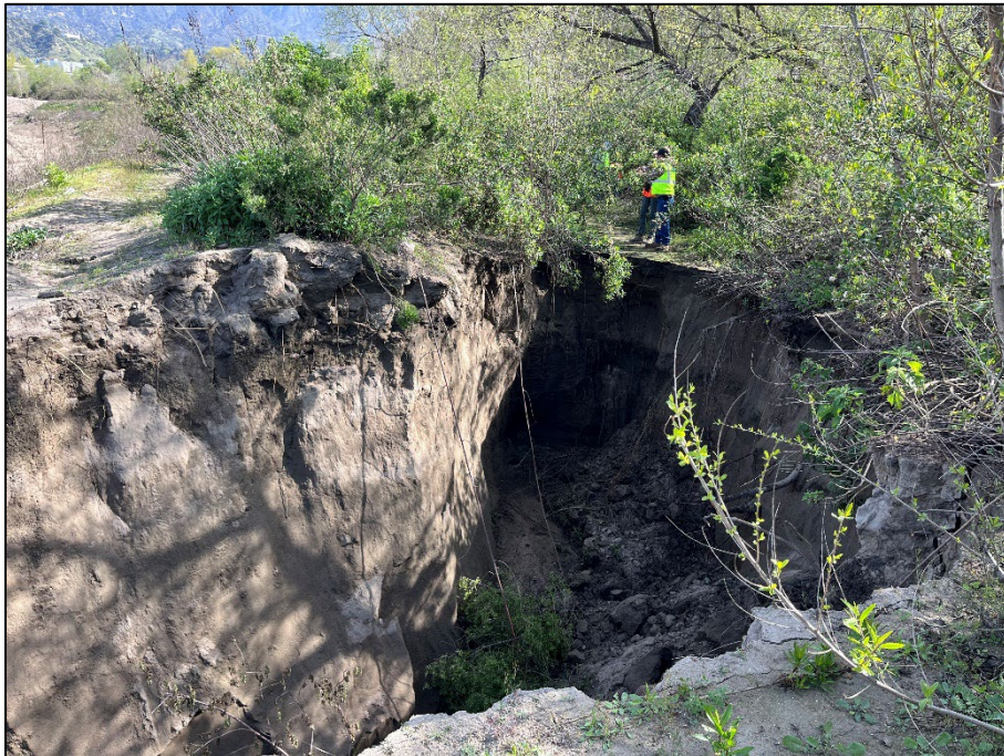
Photo 12: Erosion to Side Slopes
