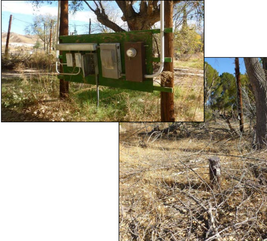
Photograph 15 - Electrical poles and panels (upper left) and electrical hookups, possibly for RVs, were observed on the western parcel.
