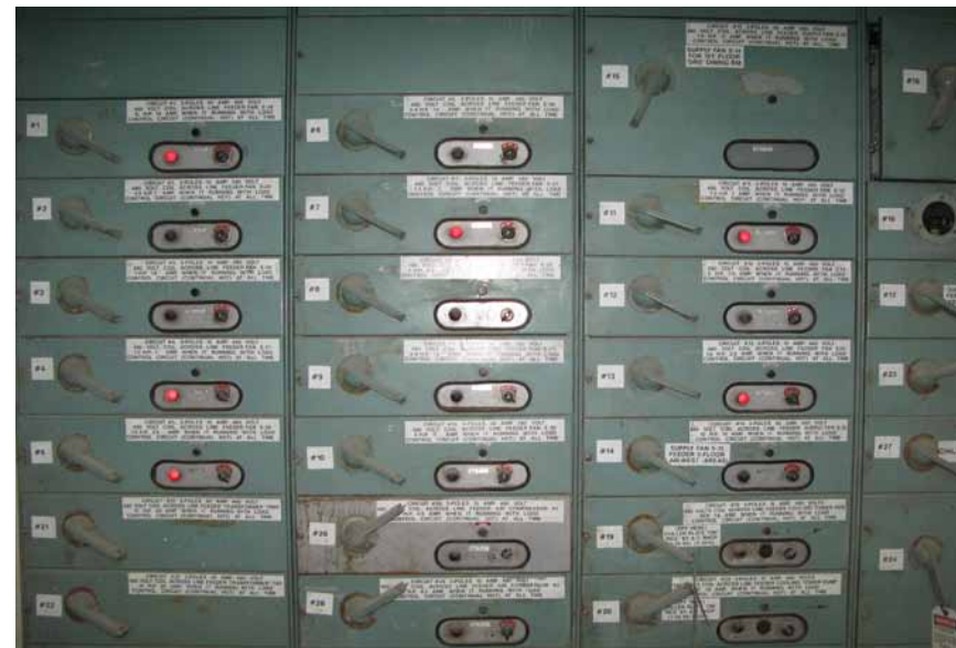
Outdated electrical gear in Main Hospital
