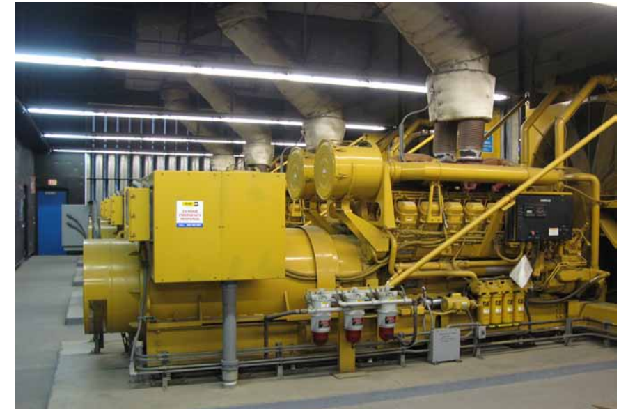
Central plant generators
