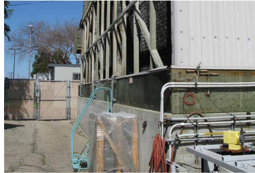
Campus mechanical equipment
