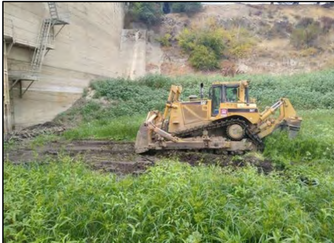
Photo Number: 3 Location: South Side of the Reservoir Near Dam Wall Description: Dozer Clearing/ Removing Vegetation
