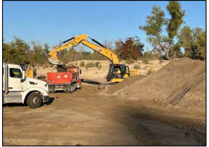
Photo Number: 14 Location: North Side of the Reservoir Description: Excavator Loading Sediment into Truck
