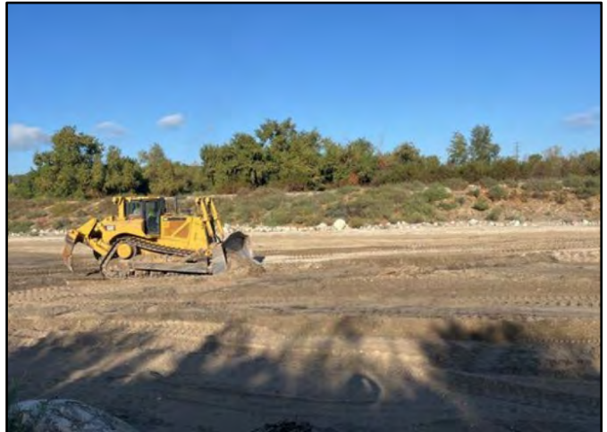
Photo Number: 4 Location: North Side of the Reservoir Description: Dozer Clearing/ Removing Vegetation
