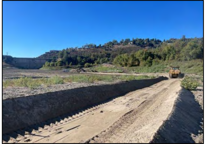
Photo Number: 10 Location: Along West Side Edge of Reservoir Description: Bulldozer Channeling
