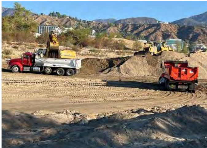
Photo Number: 11 Location: North Side of the Reservoir Description: Bulldozer Compiling Sediment for Excavator
