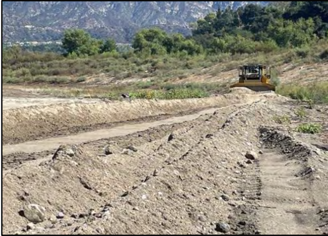
Photo Number: 9 Location: Along East Side Edge of Reservoir Description: Bulldozer Channeling
