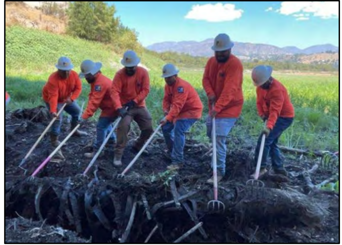
Photo Number: 2 Location: South Side of the Reservoir Near Dam Wall Description: Crew Removing Debris
