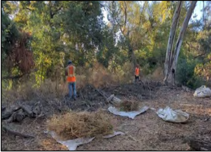
Photo Number: 27 Location: DG-4 Area Description: Crew Hand pulling Weed/ Weed Abatement
