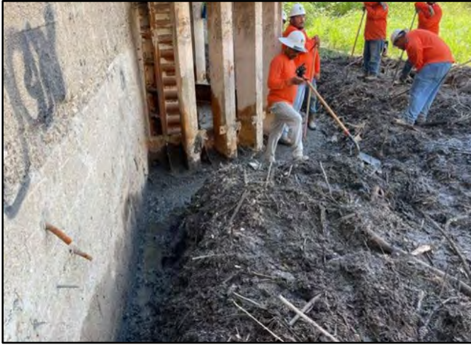
Photo Number: 1 Location: South Side Near Dam Wall and Gate Description: Crew Removing Debris from Dam Wall and Gate
