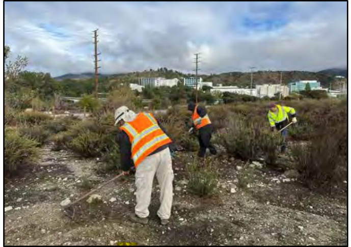
Photo Number: 32 Location: DG-4 Area Description: Redefining Irrigation basins and removing nonnatives
