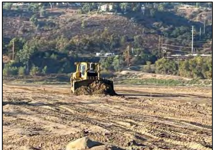
Photo Number: 12 Location: South Side of the Reservoir Description: Bulldozer Grading Reservoir
