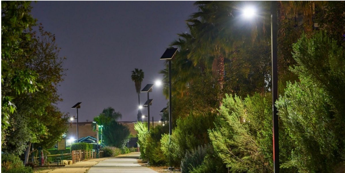
Figure 10-32. Solar lighting fixture on Whittier greenway
