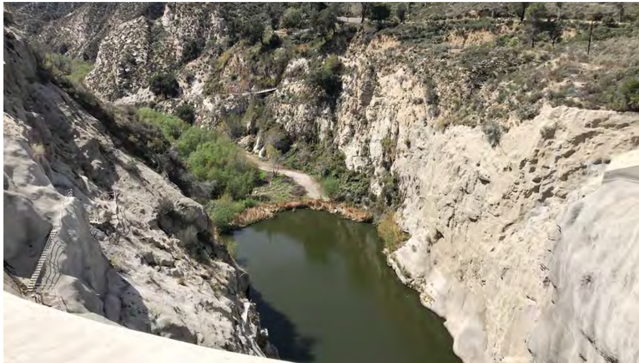
Photo 3: Photo depicts plunge pool west of BTR dam structure, followed by Big Tujunga Creek and access road, looking south.
